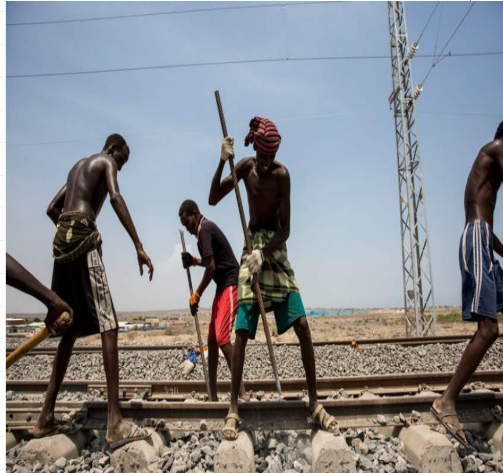
Workers maintain and check the Addis Ababa-Djibouti railway during a trial run in Addis Ababa, Ethiopia, on Sept. 28, 2016. Days later, after four years of construction and funding by the Chinese, it opened to become Africa's first cross-border electrified railway. ImagineChina/AP
